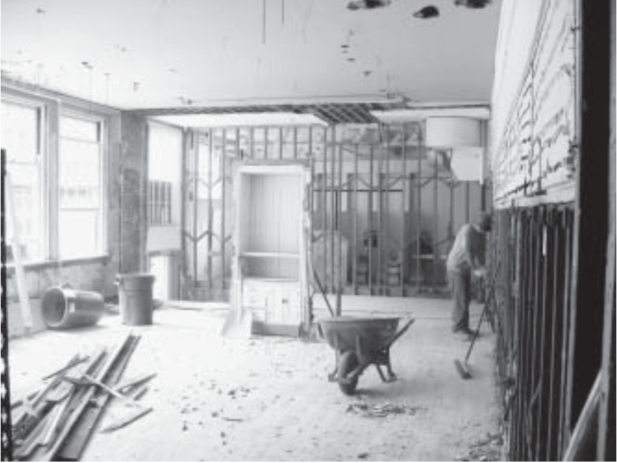
Walls removed to studs looking at the new home of the Treasurer.
