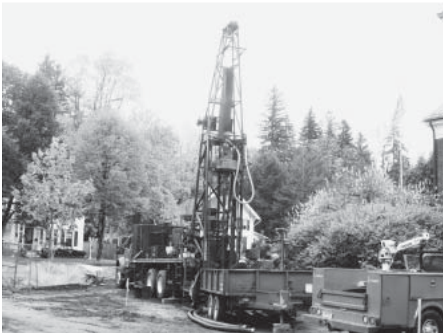
Drilling of a Geothermal well. This well is just one of three that will provide heat and air conditioning to the building.
